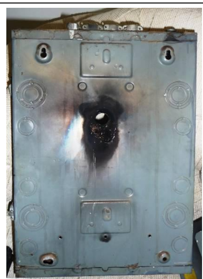
Fig. 9. Burned Panel Rear Photo courtesy SCM Engineering, © 2012. Used with permission.
