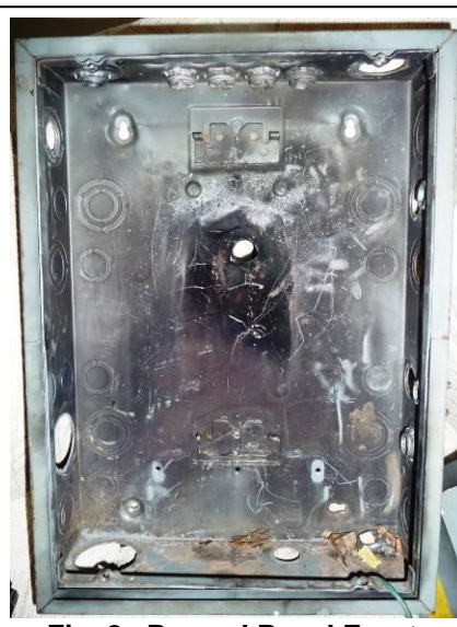
Fig. 8. Burned Panel Front Photo courtesy SCM Engineering, © 2012. Used with permission.
