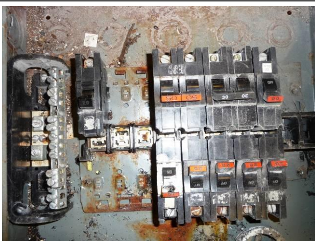
Fig. 10. Corrosion and “Burn” Marks on a Stab-lok Panel
